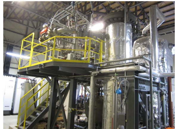
Figure 9: The Kalina power generation system using hot spring fluid at Matsunoyama.
