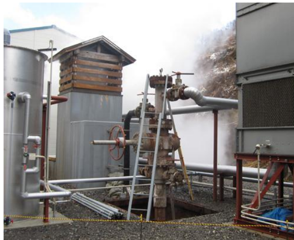
Figure 5: Wellhead of Takanoyu#3.
